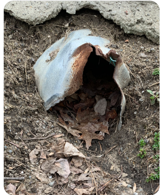
Damaged storm sewer culvert (Giffels Webster)
