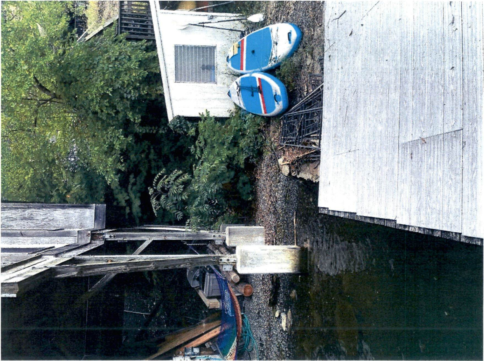
View along lakeshore property line between 281 and 290 Bill George Rd. - North edge of concrete pad shown deteriorating.
