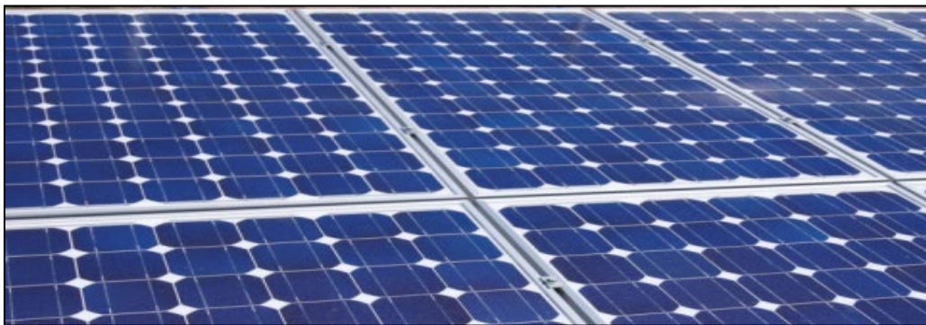
Figure 11. Module Spacing Gaps
