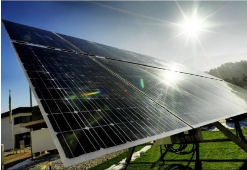
Solar panel showing solar glare
