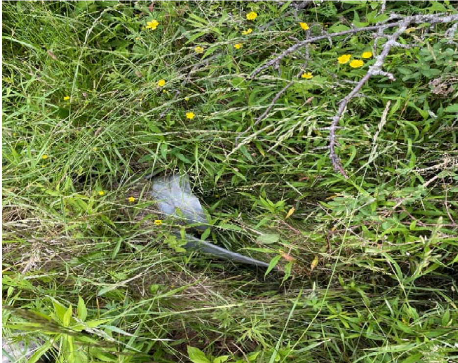
Photo 12. View looking at a pipe culvert feeding water from the 'A/B' flagged wetland towards the 'C/D' wetland.
