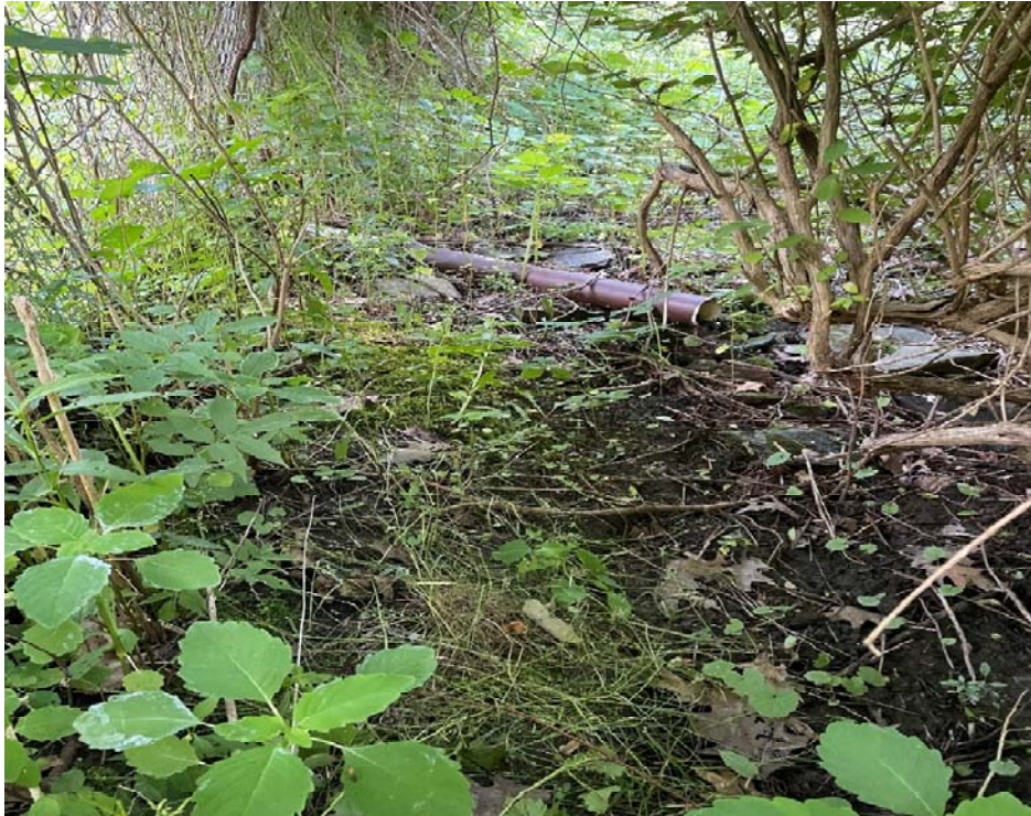
Photo 10. View facing east looking at a pipe culvert feeding water into the site from the northern boundary of the inspection area.
