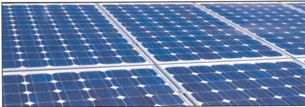
Figure 11. Module Spacing Gaps
