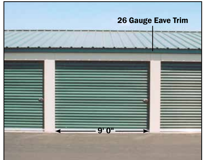
a. The typical 10' bay utilizes a 9'0" wide door, and a typical 12'0" wide bay uses an 11'0" wide door.
