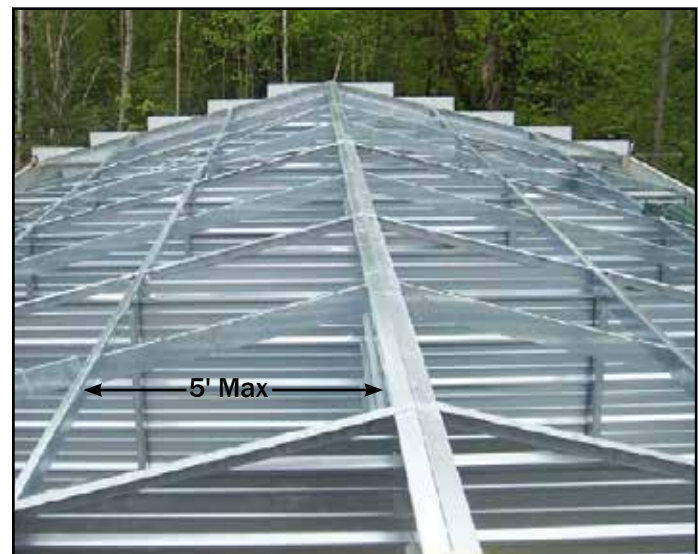
b. The interior structure has 5' purlin spacing standard, in some high snow load areas closer purlin spacing may be required.
