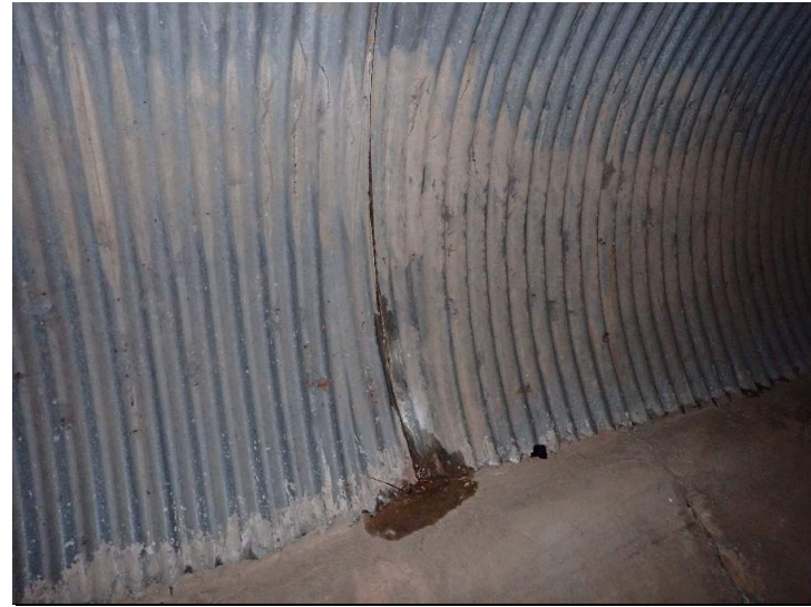
MIDDLE SEAM WITH MINOR LEAKAGE, SOUTH SIDE
