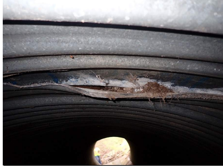
FILL VISIBLE AT TOP OF MIDDLE SEAM
