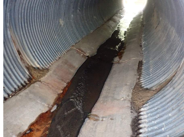
BOTTOM OF CMP LINED WITH CONCRETE, FAIR CONDITION
