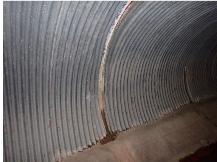
EAST SEAM WITH MINOR LEAKAGE AT SOUTH SIDE
