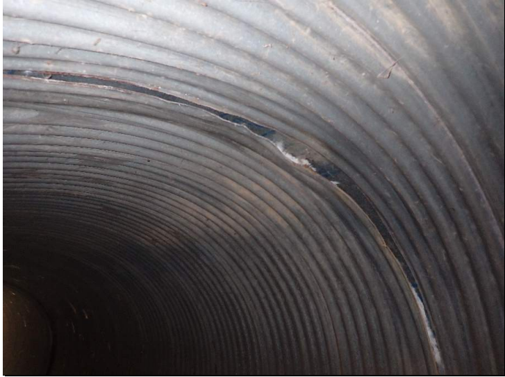
POSSIBLE DAMAGED END OF MIDDLE SEAM, NORTH SIDE
