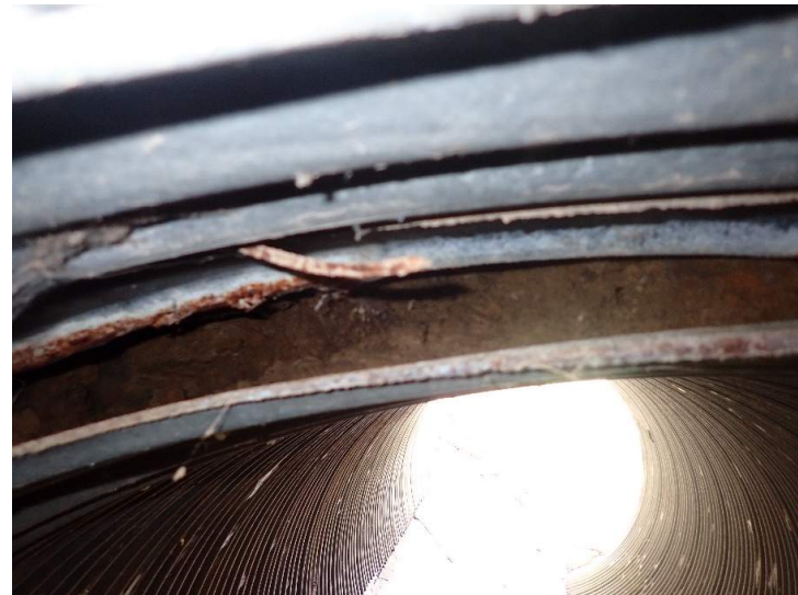
WEST SEAM OPEN APPROX. 1.25" AT TOP, FILL VISIBLE
