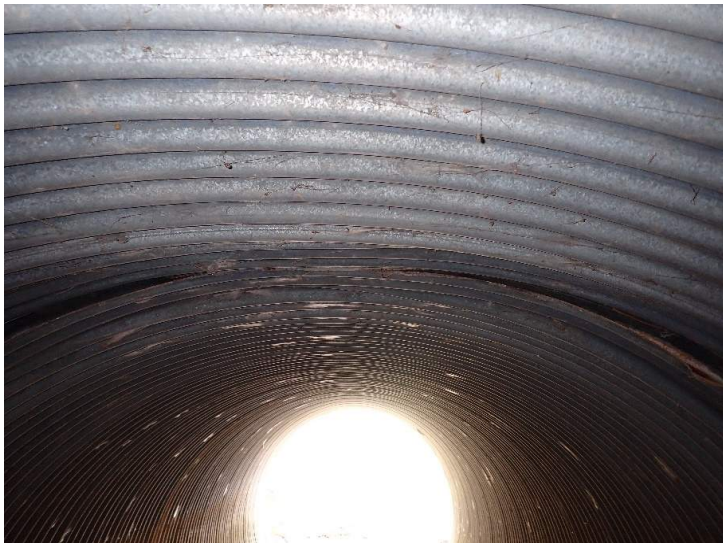
VISIBLE DEFLECTION IN CEILING AT WEST SEAM
