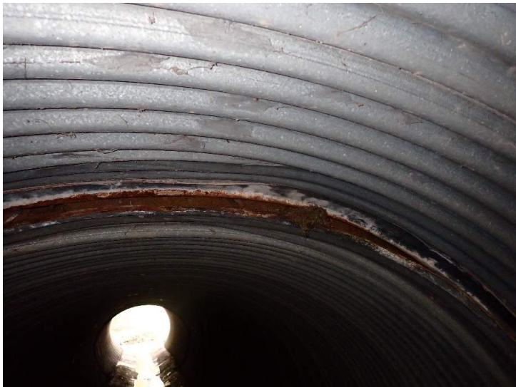
EAST SEAM OPEN 1.25IN, VISIBLE FILL
