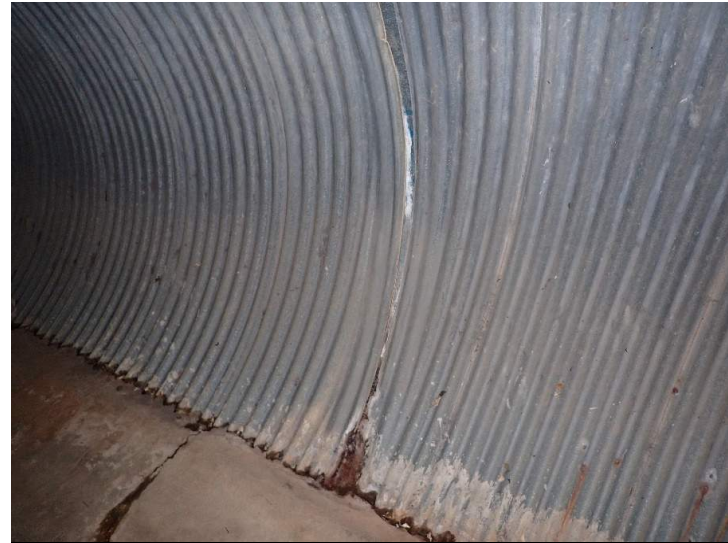
MIDDLE SEAM WITH MINOR LEAKAGE, NORTH SIDE
