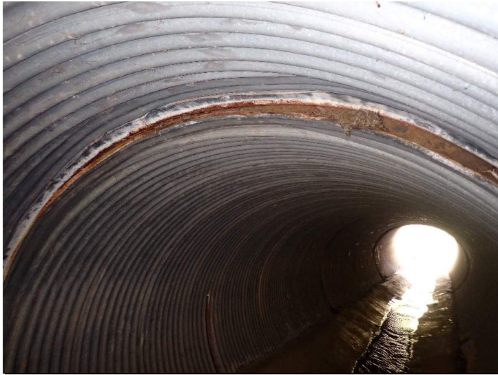
EAST SEAM OPEN 1.25IN, VISIBLE FILL
