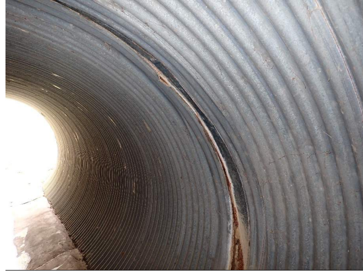
WEST SEAM, NORTH SIDE OPEN APPROX. 1IN AT CORNERS
