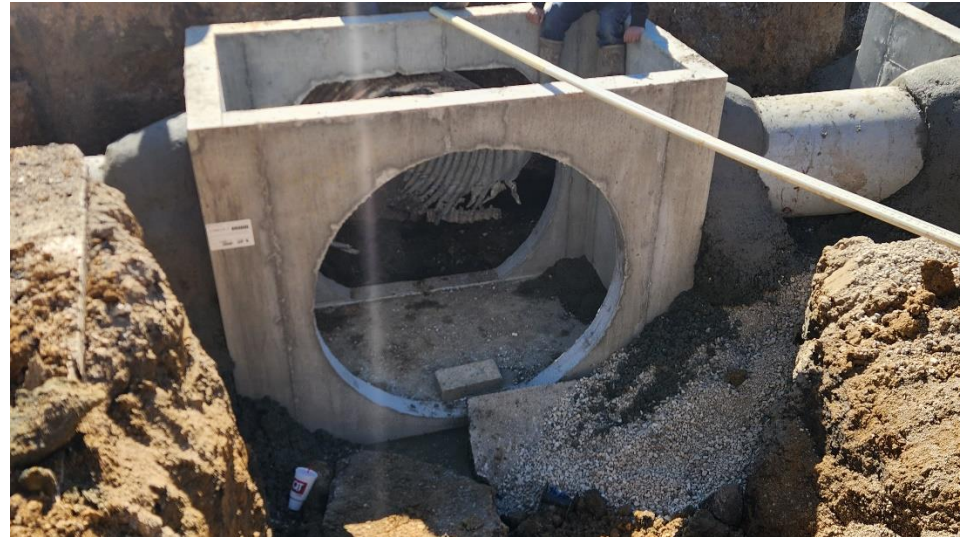
Photo #4 – Junction Box JB-A2 (looking south)
