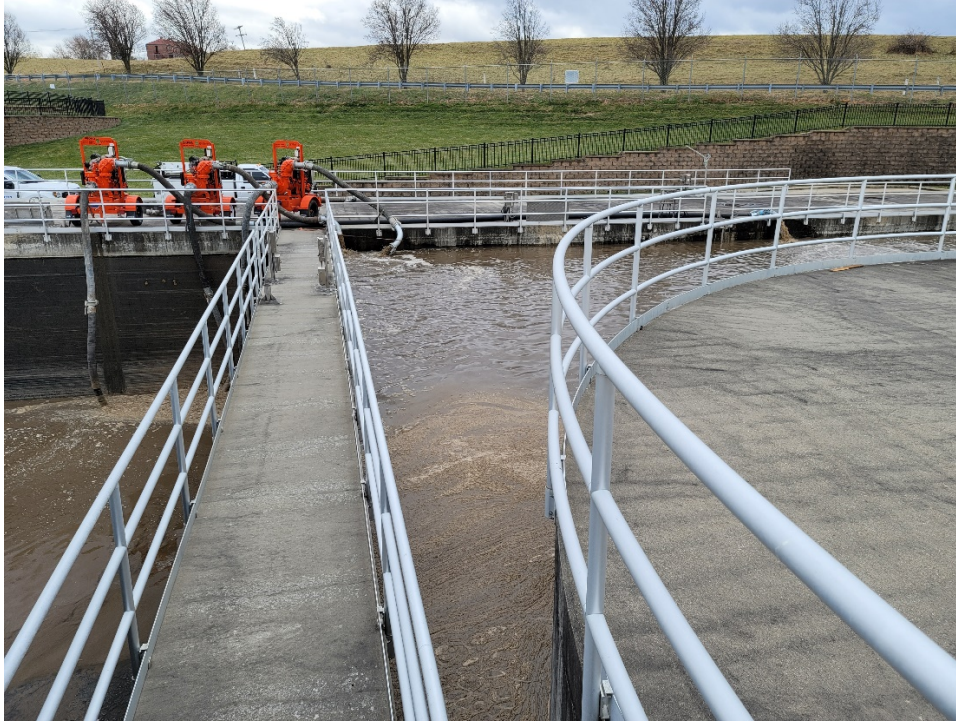
Three 6" transfer pumps draining basin D1 (left) into D2 (right)
