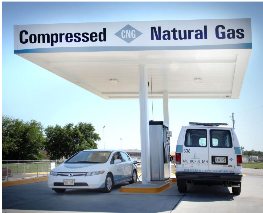
Metropolitan Utilities District (MUD) Public CNG Station Omaha, NE (Source: MUD) - Left
