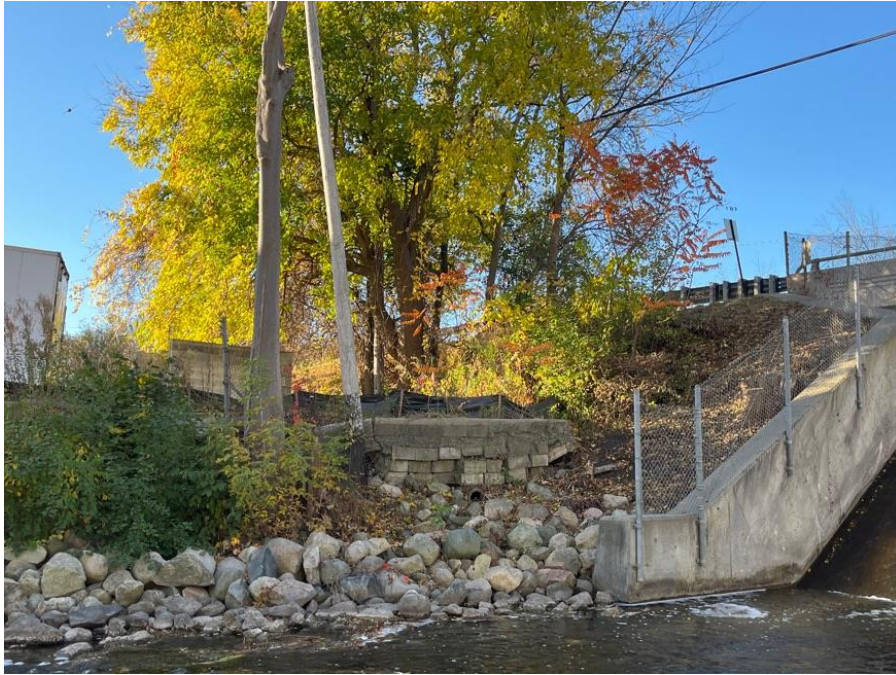
Photo #35: Embankment Downstream Slope. Right slope shown. Issue: Trees and Brush, Ground Cover, Action: Monitor, Maintenance
