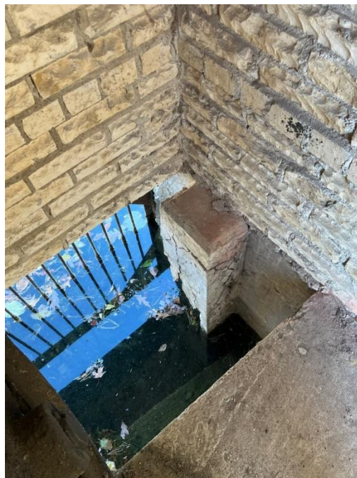
Photo #24: Auxiliary Spillway Headwall. Note deteriorating concrete column. Issue: Deteriorating Material, Action: Monitor, Maintenance
