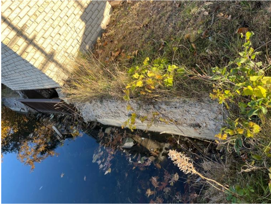
Photo #21: Auxiliary Spillway Headwall. Issue: Deteriorating Material, Action: Monitor, Maintenance
