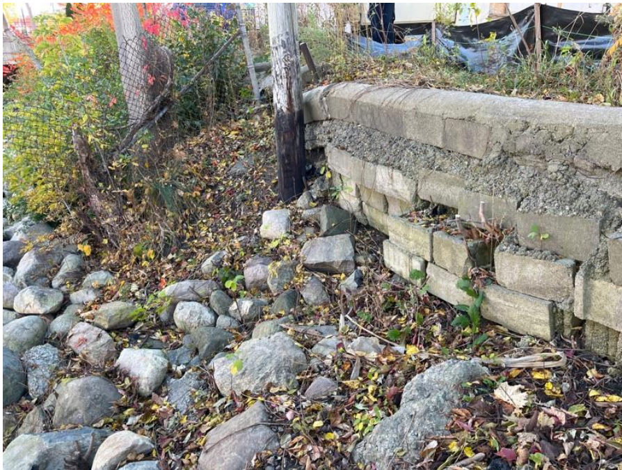
Photo #34: Embankment Downstream Slope. Deteriorating concrete block retaining wall shown with drain outlet on right downstream slope.
