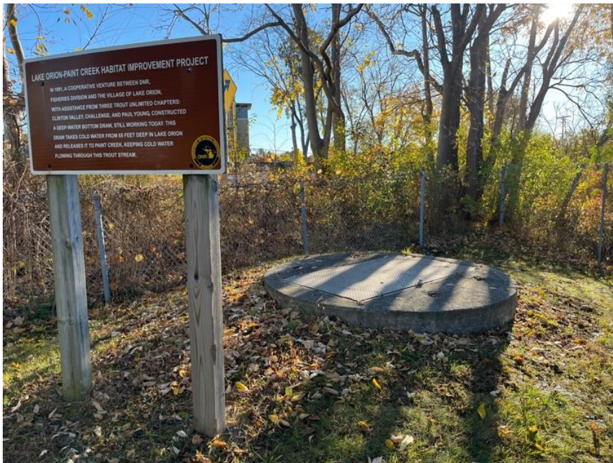
Photo #25: Embankment Upstream Slope. Cold water inlet at the park immediately north of the dam.
