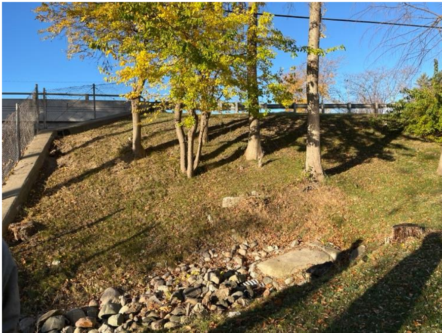
Photo #36: Embankment Downstream Slope. Left slope shown. Issue: Trees and Brush, Action: Maintenance
