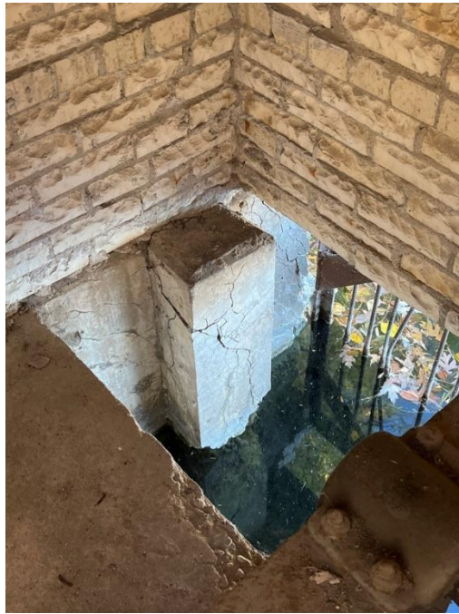
Photo #23: Auxiliary Spillway Headwall. Note deteriorating concrete column. Issue: Deteriorating Material, Action: Monitor, Maintenance
