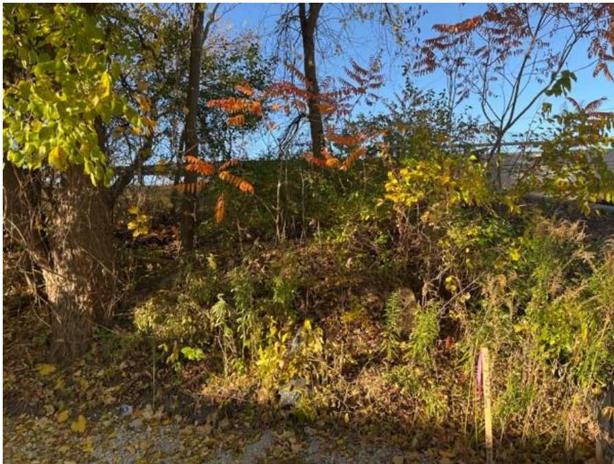
Photo #38: Embankment Downstream Slope. Right slope shown. Issue: Trees and Brush, Action: Maintenance
