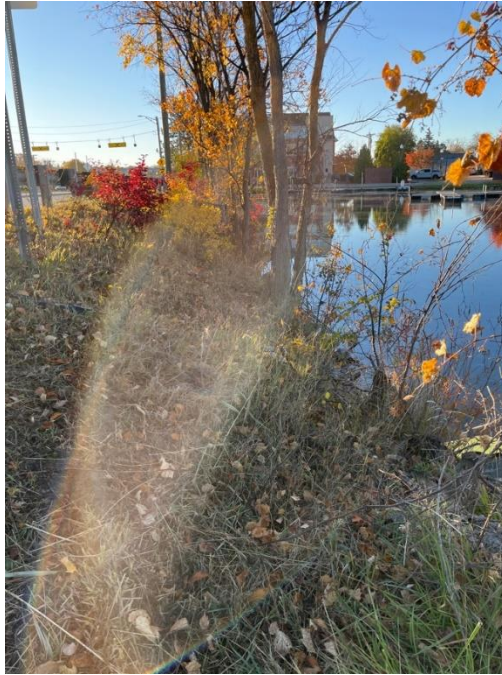
Photo #29: Embankment Upstream Slope. Right slope shown. Issue: Trees and Brush, Action: Maintenance
