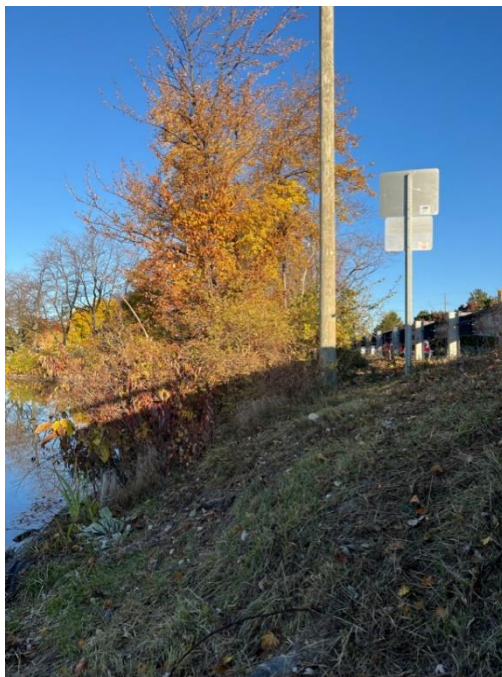
Photo #28: Embankment Upstream Slope. Left slope shown. Issue: Trees and Brush, Action: Maintenance
