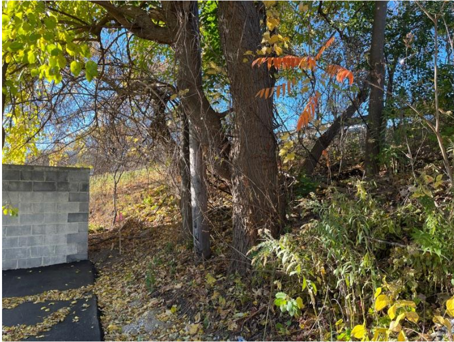
Photo #39: Embankment Downstream Slope. Right slope shown. Issue: Trees and Brush, Action: Maintenance
