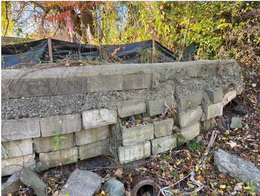
Photo #33: Embankment Downstream Slope. Deteriorating concrete block retaining wall shown with drain outlet on right downstream slope.
