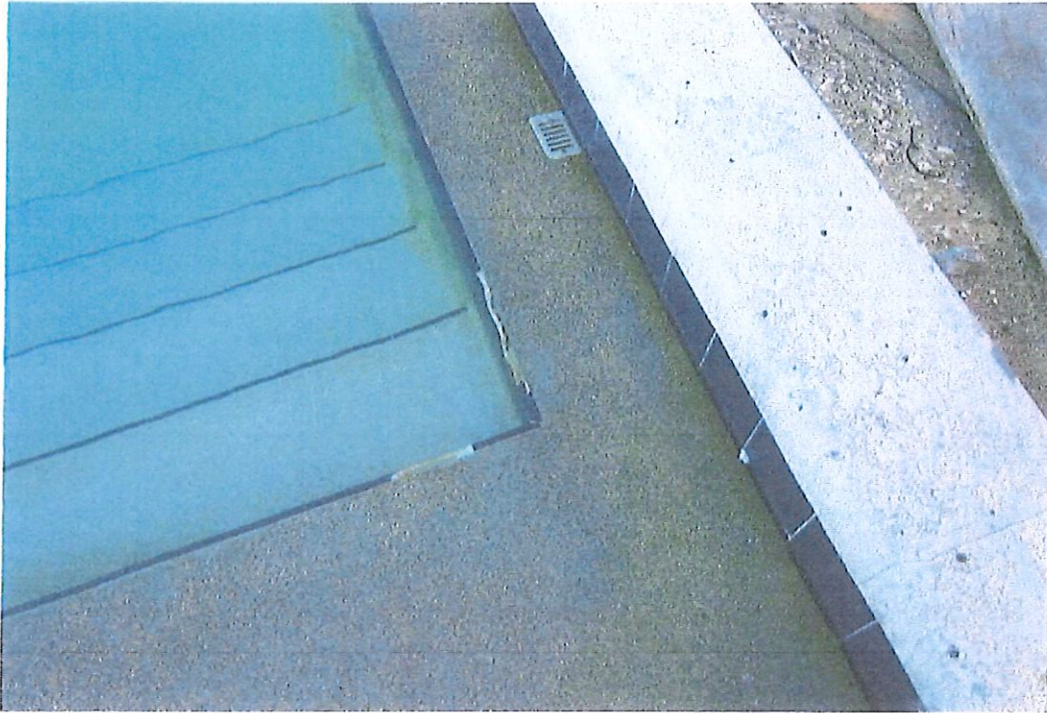
EXHIBIT 7. VIEW OF MISSING BULLNOSE TILE (REFERENCE EXHIBIT 6.)
