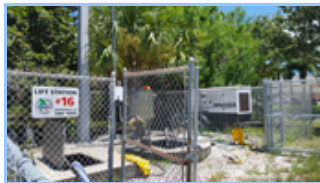
Local Sewer Lift Station
