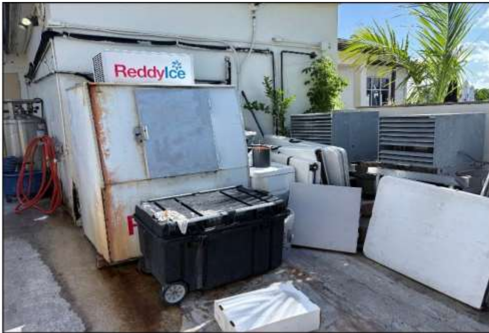
Ice Maker & Walk In Box & Freezer Compressors
