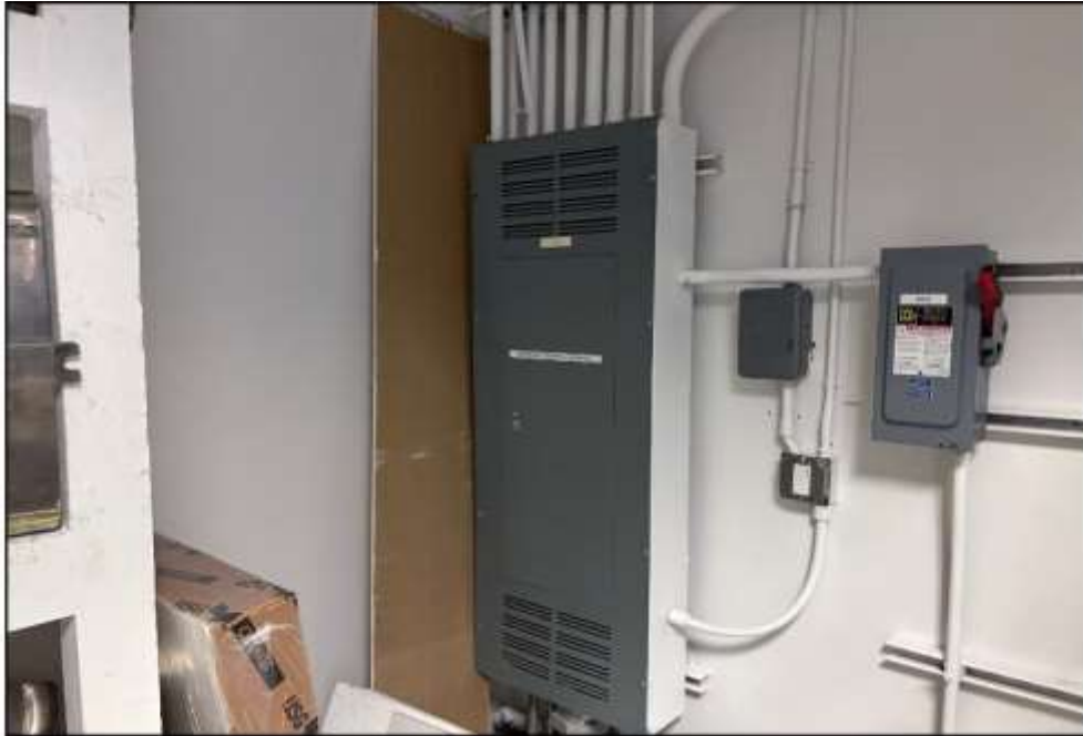
Main Electric Distribution Panel
