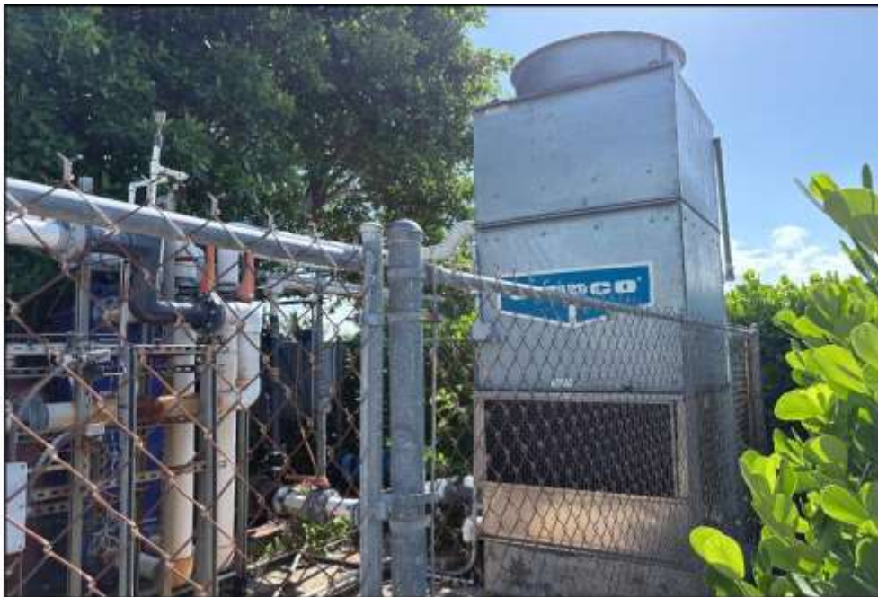
Air Conditioner Compressor
