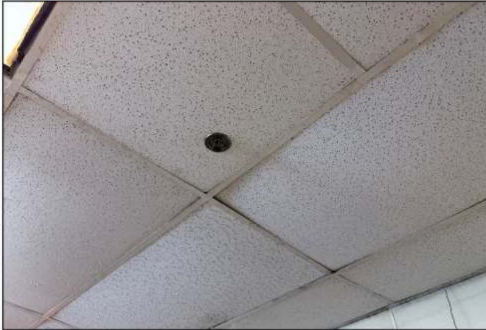
Typical Sprinkler Head
