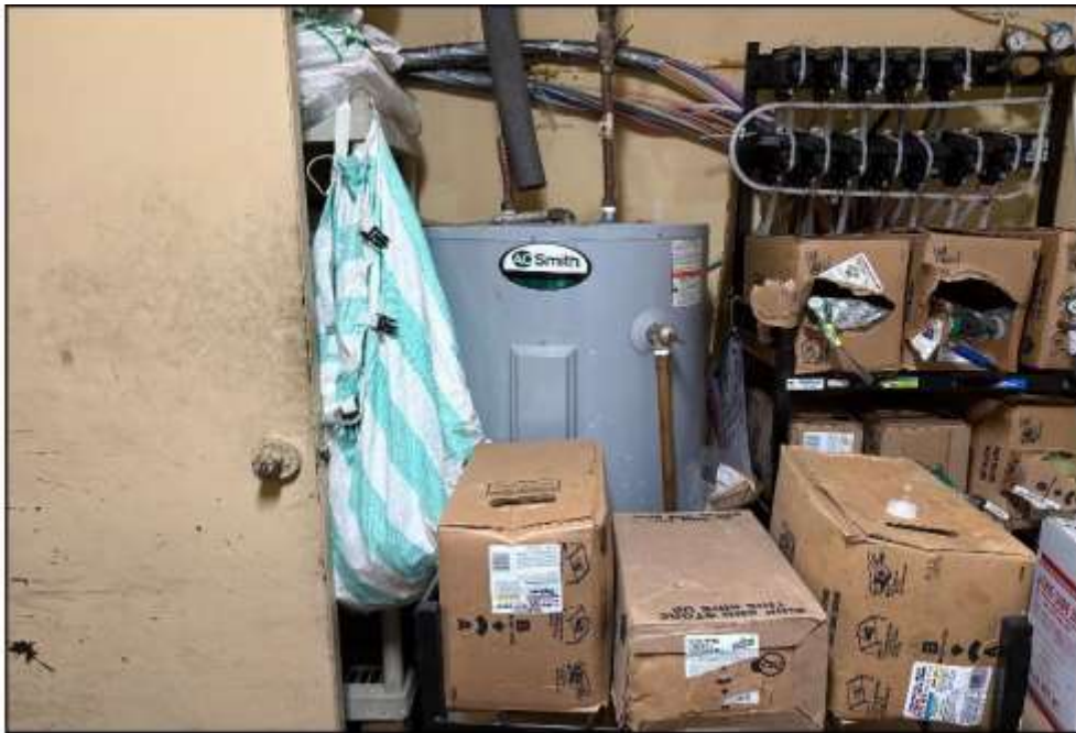
Hot Water Heater
