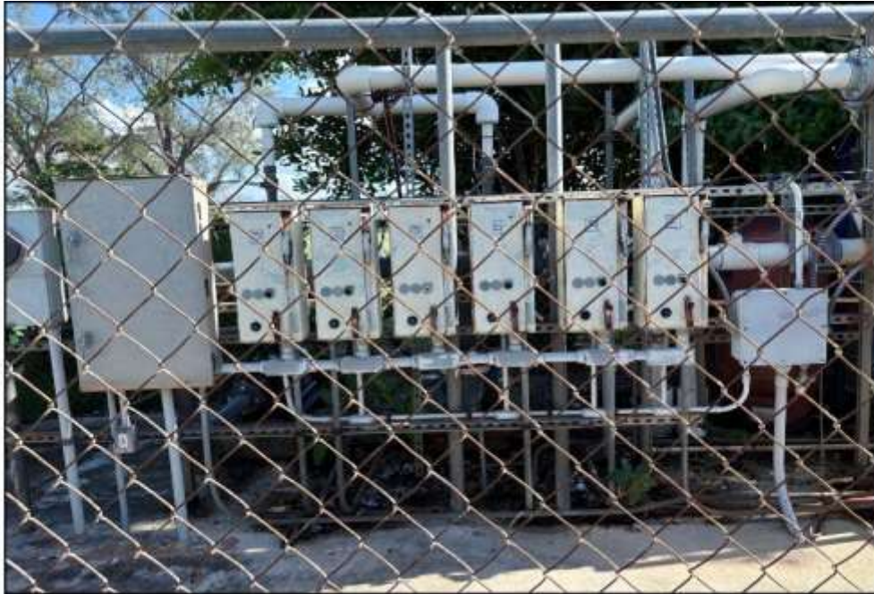
Breaker Panel for Central Air Unit
