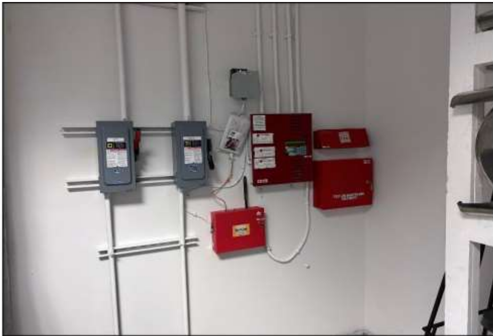
Fire Suppression and alarm systems
