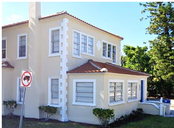
Example: 331 South Federal Highway Before: Mixture of original wood double-hung windows and replacement awning windows
