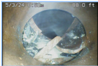
Local Sewer Collection system Pipe
