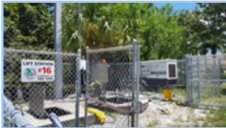
Local Sewer Lift Station
