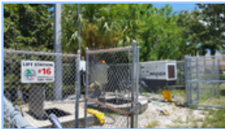
Sewer Pump Station
