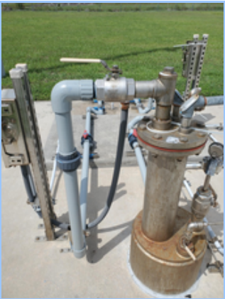
Dual Zone Monitoring Well
