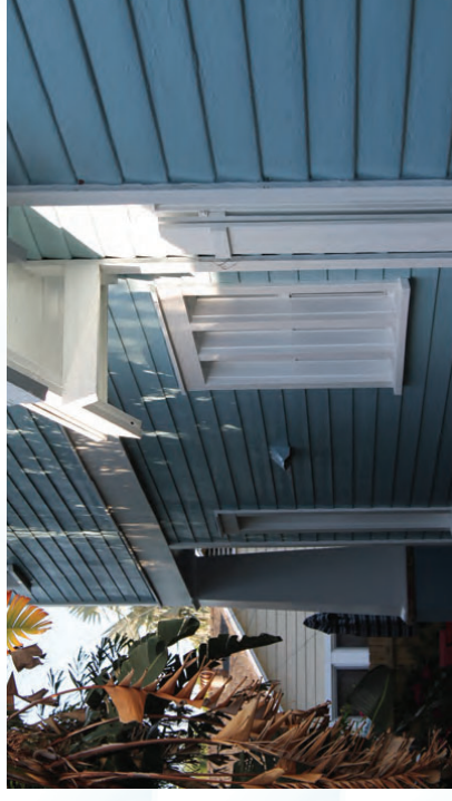
This image shows a historic structure in the foreground with a new two-story addition beyond.
