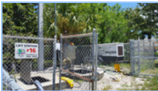
Local Sewer Lift Station
