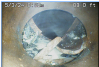
Local Sewer Collection system Pipe
