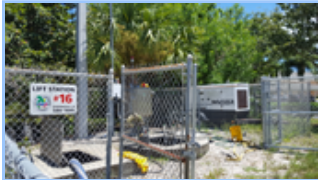
Sewer Pump Station
