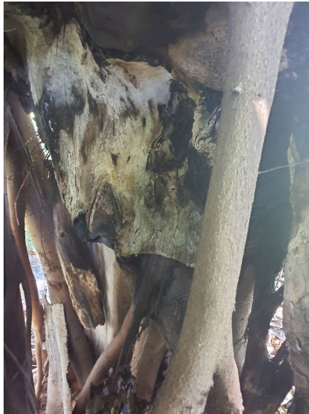
Photo 8. View of trunk damage on the north side of Tree 105, facing north. Note that this wound is towards the inside of the trunk; the outer portion of the trunk (which provides a greater influence on structural integrity in comparison to the inner portion) remains intact.
