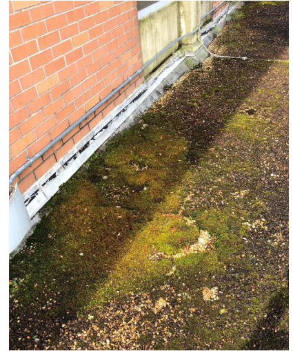
Organic growth on roof membrane
