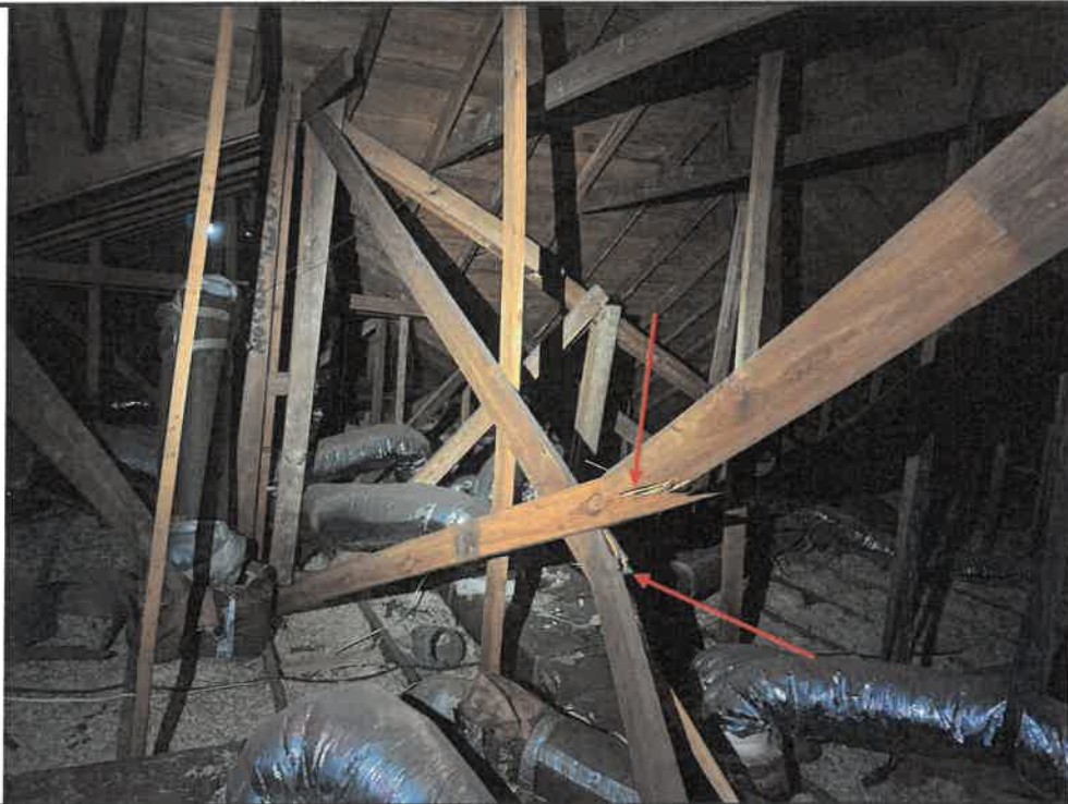
Photo 5: Broken x-bracing between Truss-A and Truss-B
