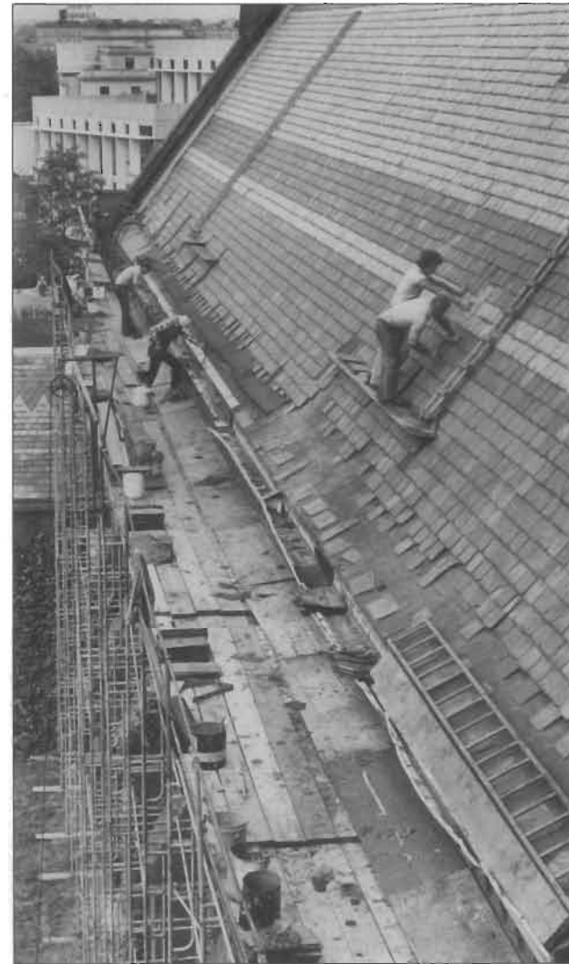
Workmen are in the process of removing deteriorated roofing slates and replacing them with new matching slates.
