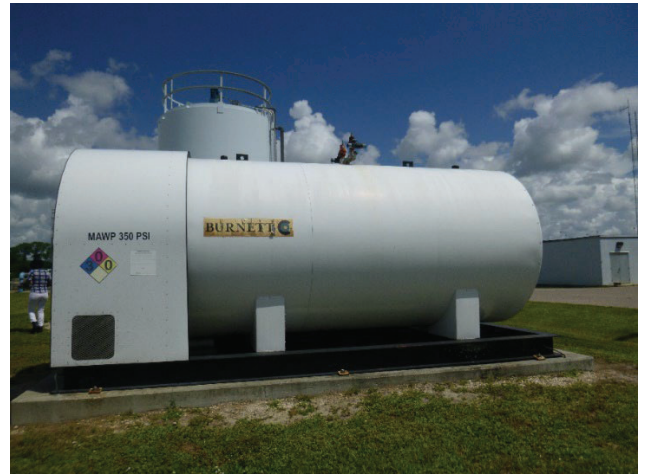
Photo 16: View of CO2 storage Tank and power panel.
