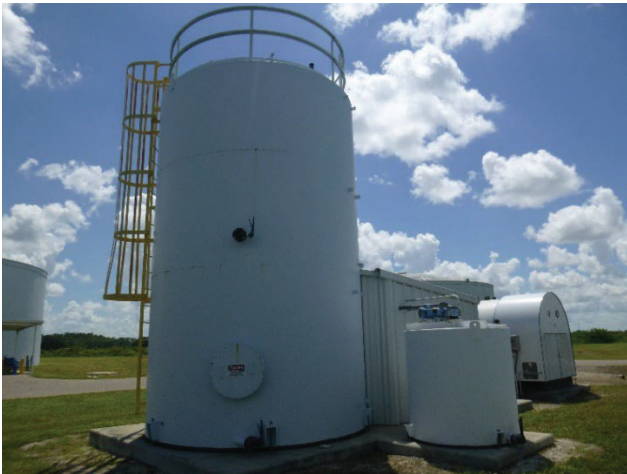
Photo 15: View of 16,000-Gal lime slurry storage tank and control panel.
