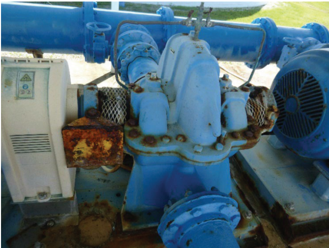
Photo 9: View of corrosion on pipes.
