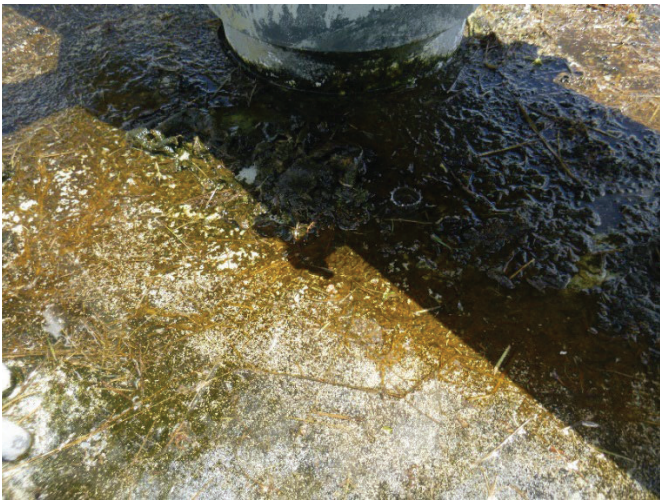
Photo 19: View of wet concrete from leak at well casing.
