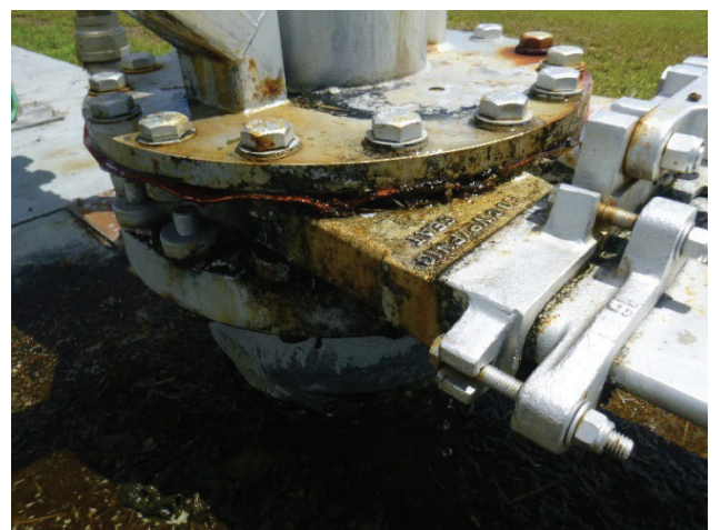
Photo 18: View of well casing leaking.
