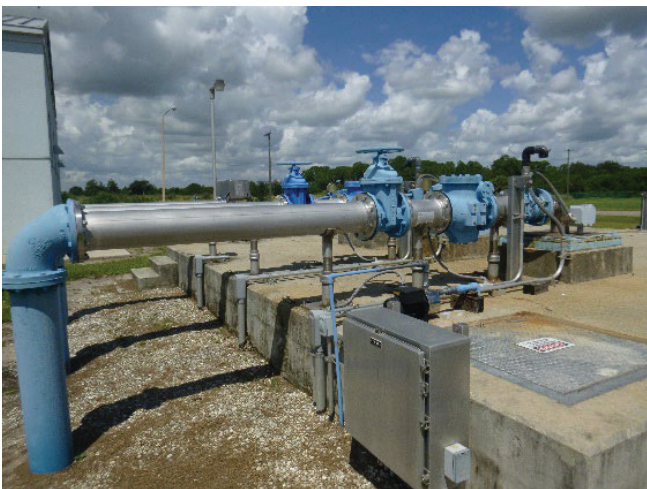
Photo 5: View of clearwell and transfer pumps.
