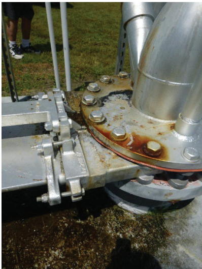
Photo 20: View of leaking well casing.
