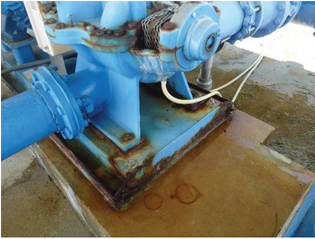
Photo 13: View of corrosion at base of pump.
