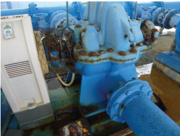
Photo 11: View of corrosion on pipes.
