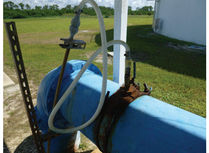
Photo 10: View of corrosion on pipes.
