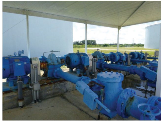
Photo 8: View of high service pumps.
