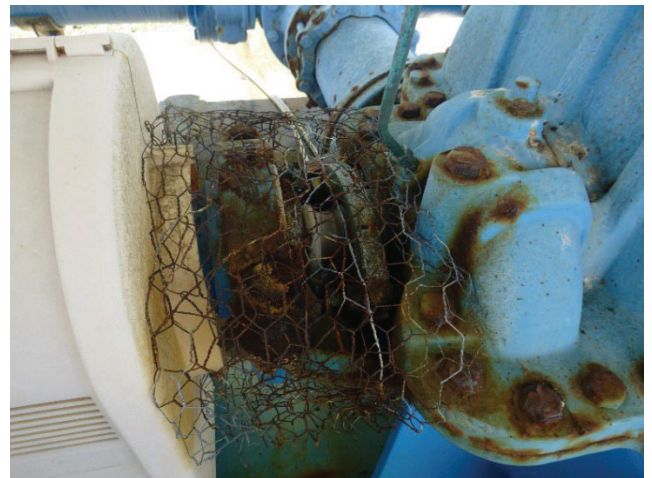
Photo 12: View of corrosion on pipes.
