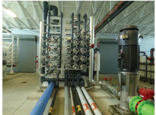
Photo 2: View of second train in RO system.
