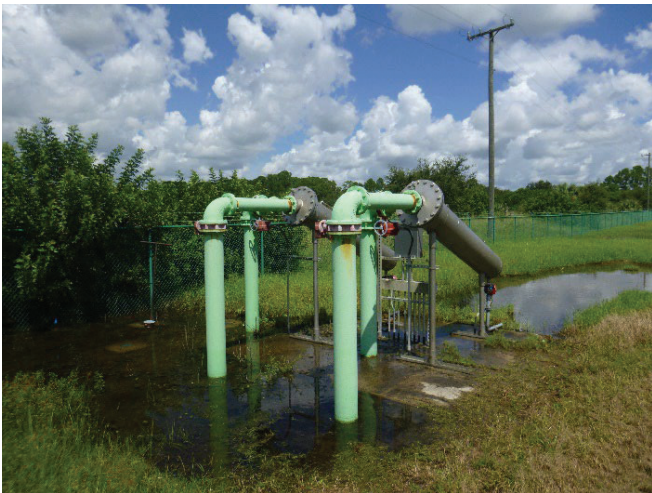
Photo 3: View of sand separator.
