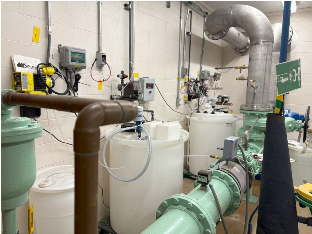
Chemical Feed Equipment Installed
