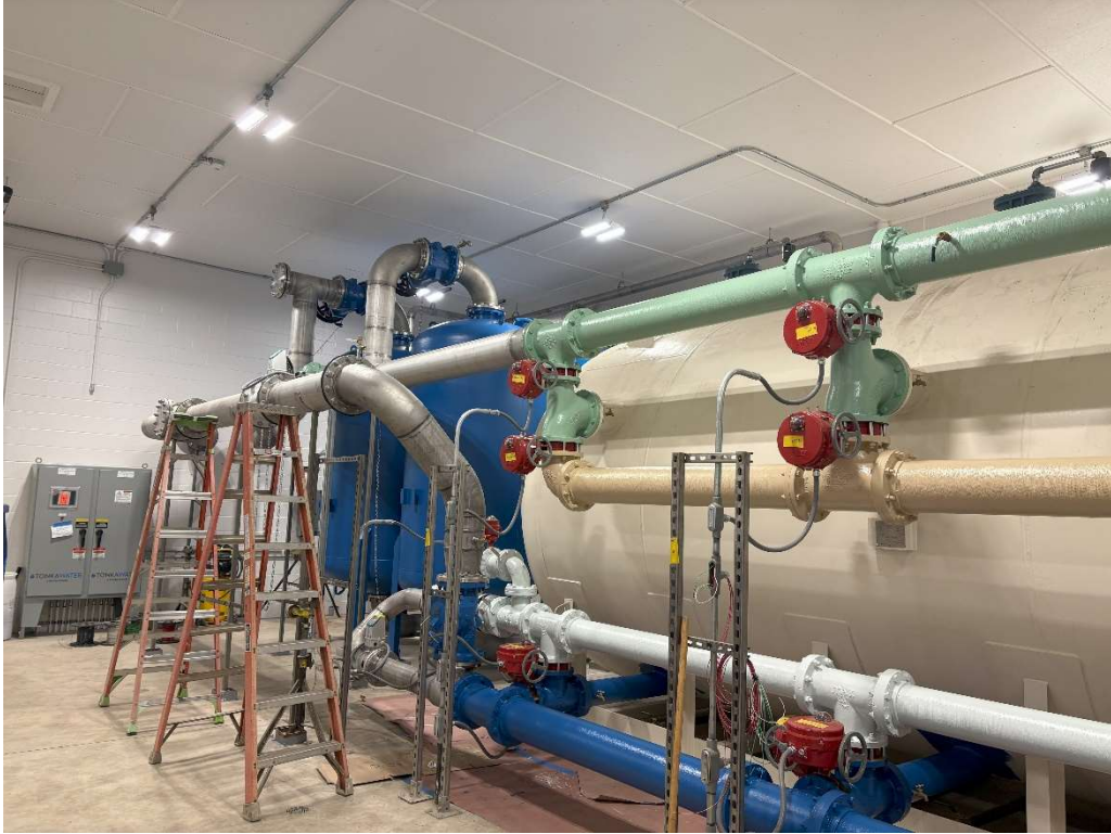
Coatings on Vessels and Piping
