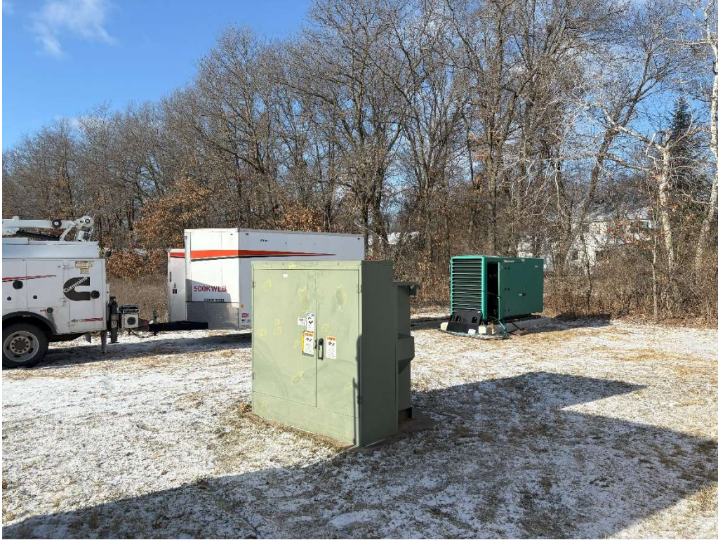
Generator Load Bank Testing
