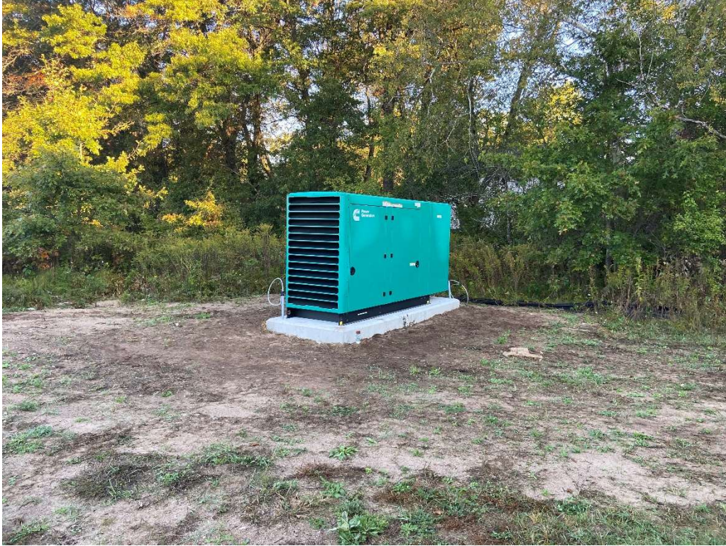
Generator Installed on Pad.
