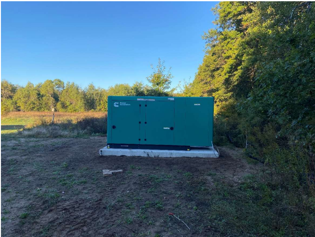
Generator Installed on Pad.
