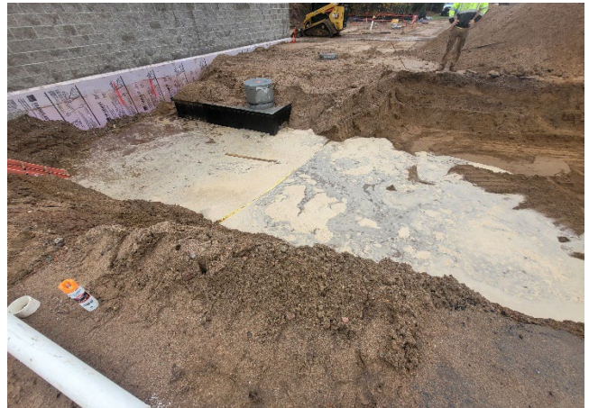
Water Filled Excavation Hole after WM Break
