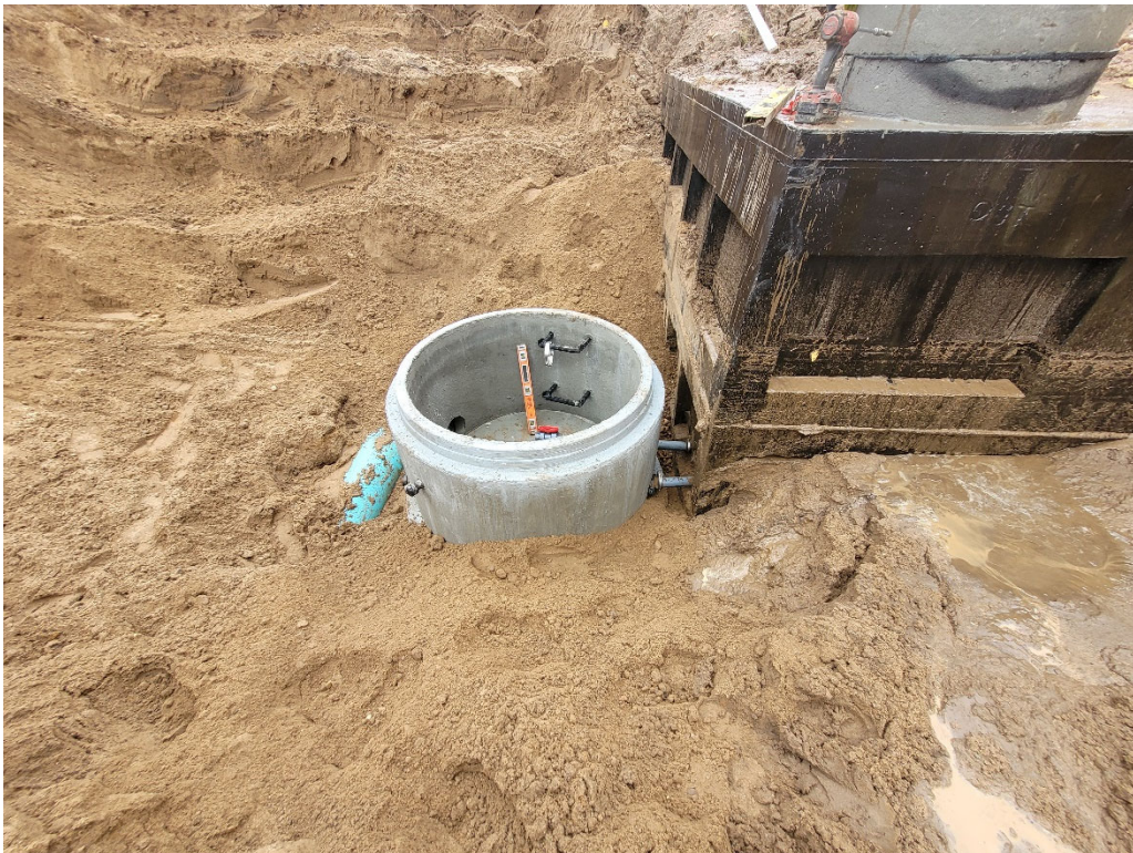
Underground backwash tank discharge manhole
