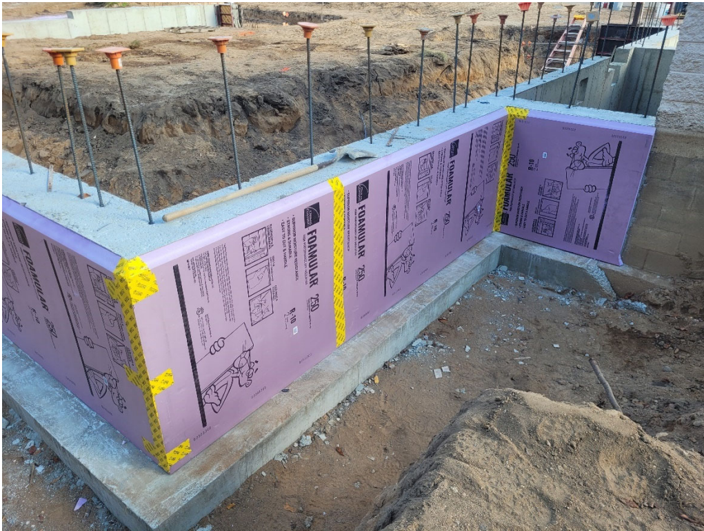
Insulated frost walls at northeast corner of Well #2
