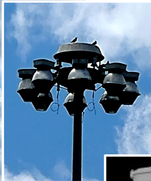
High pressure sodium fixtures
