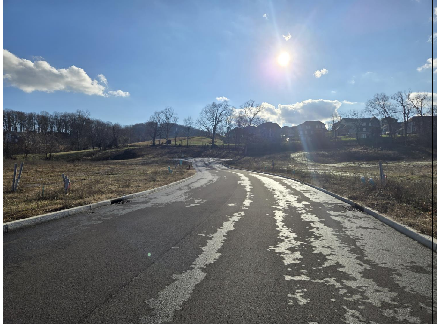
Saint Andrews Garth Phase 3 Western View
