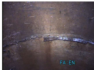
Manhole Defect Photos:
