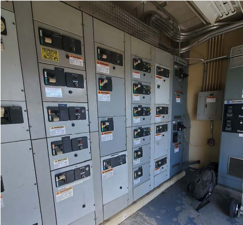
Motor Control Center (MCC) 6 – Installed in 1980 and single point of failure for critical process
