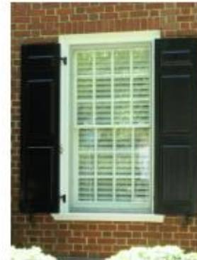
The original twelve-over-twelve, wood sash window at 1261 Watauga Street reflects the dwelling's Colonial Revival style.
