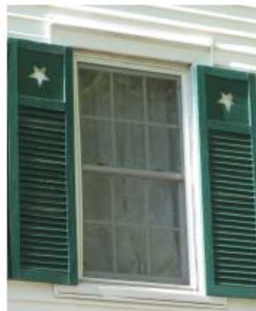
Original window shutters are used to protect windows and should be preserved and maintained (701 Yadkin Street).
