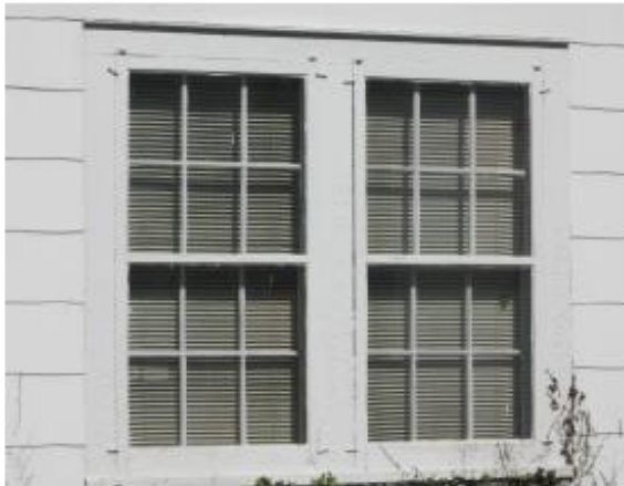
Example of an appropriate wood storm window over original six-over-six wood-sash windows (706 Yadkin Street)
