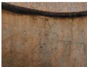
Manhole Defect Photos:
