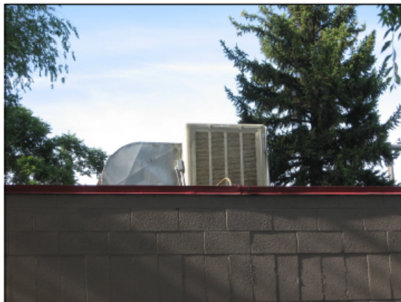
Example of a roof mechanical system set back from the street and not readily visible.
