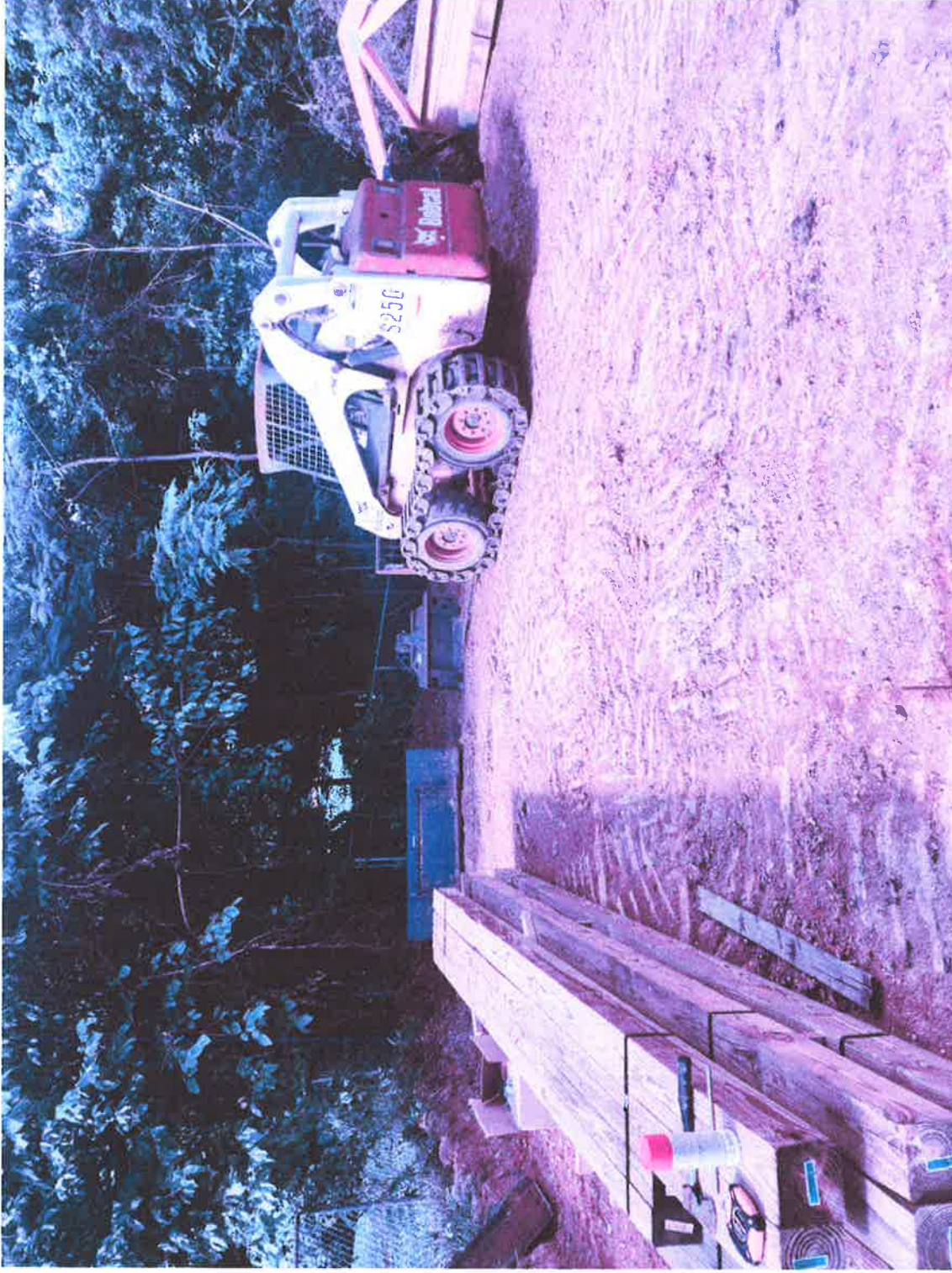
Figure 2 front left of prospective garage location, skid loaders bucket will be back of garage 15 feet from fence also showing fence line where figure one was taken from.
