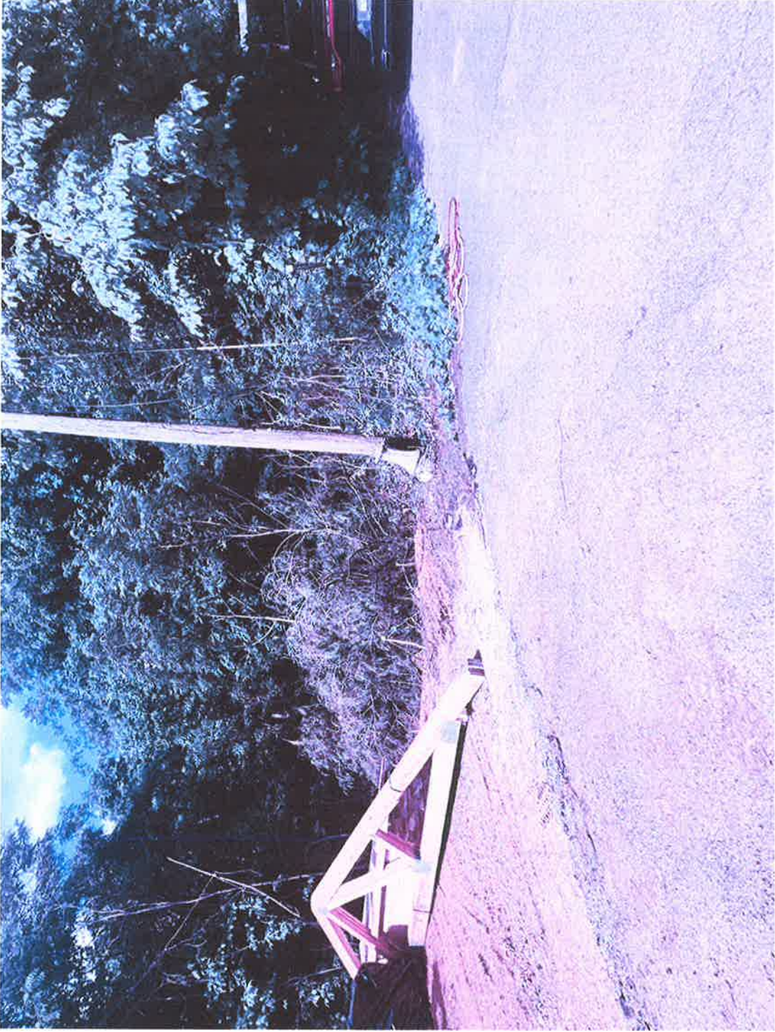
Figure 7 left front corner of garage, notice how ground level seems to disappear after tree stump
