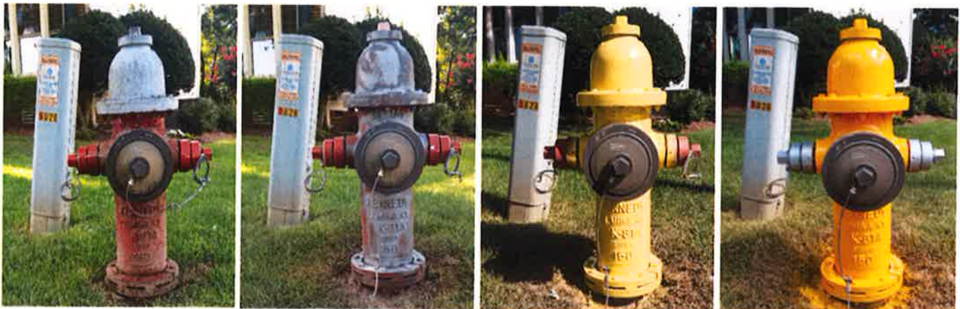
Figure 2. Raleigh NC Hydrant Painting Program
