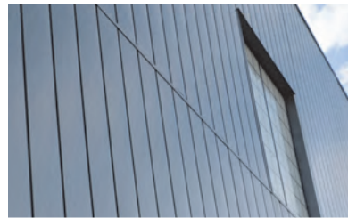
EXTERIOR FINISH 6 (EF-6): 12" WIDE METAL FLAT PANEL, VERTICAL SIDING, WESTERN STATES METAL ROOFING, MATTE PATINA
