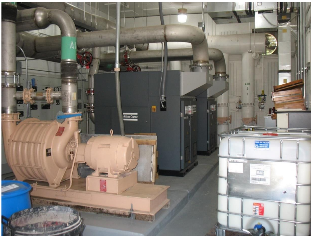
Figure 1. Existing Blower Room
