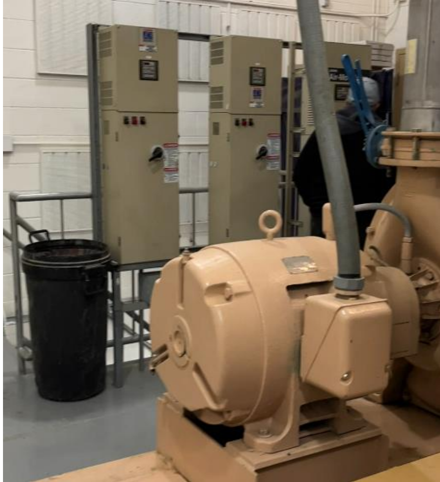
Figure 2. RAS Pump VFD Location
