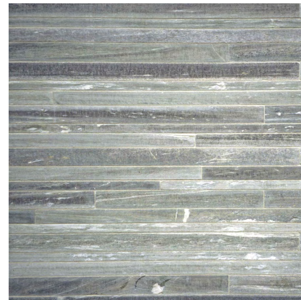
3) Stone Cladding At exterior walls
