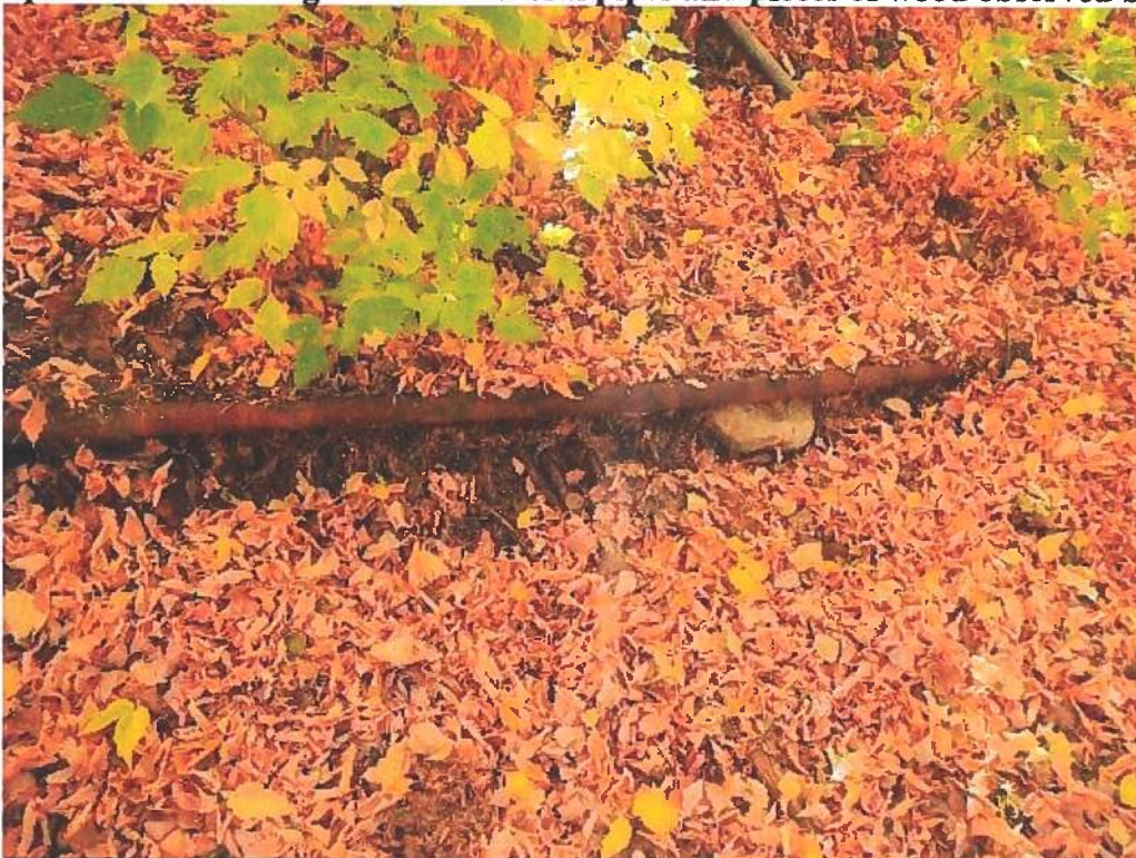
Photo 14: View of iron pipe observed along hillside outside SE side of building
