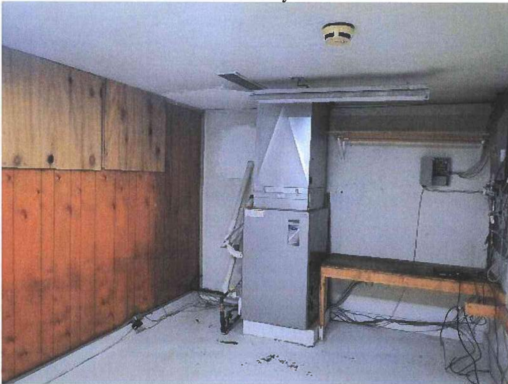
Photo 20: Gas furnace in furnace room Note: strong diesel (heating oil) odor; concrete floor
