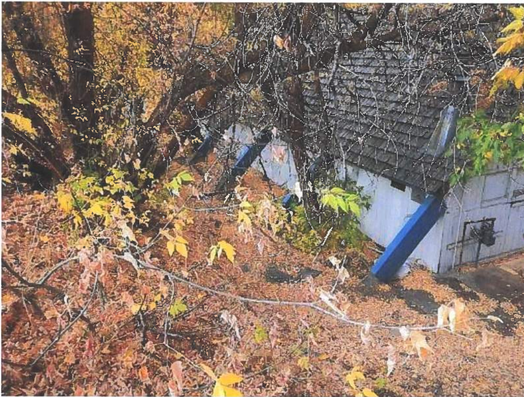
Photo 8: Looking W toward E corner of subject building Note: slope from adjacent property; gas meter; numerous leaves blocking visibility of ground
