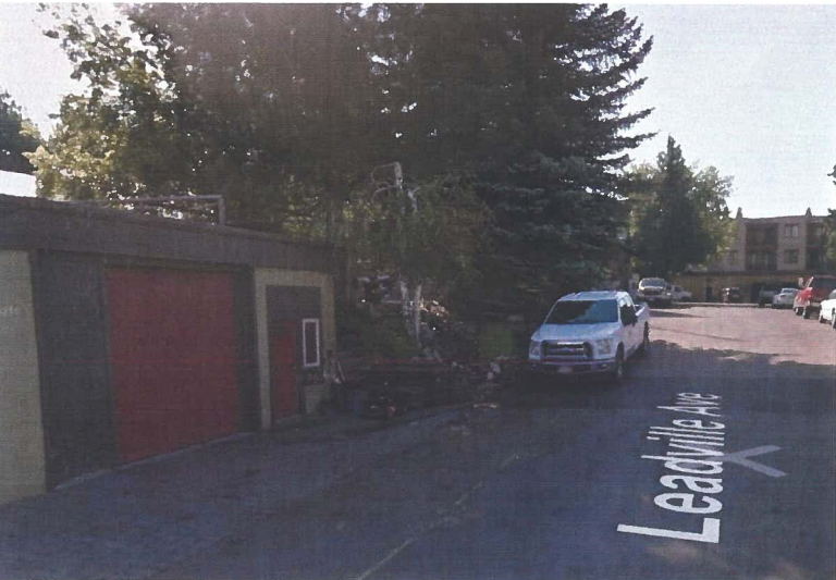
3 - Existing Site Conditions - Existing retaining wall and trees between Lots 3 & 4 has been removed. The current conditions have a 3' deep hole between the shown building and distant property line. Shown building is constructed on a zero-lot-line setback. Property line is 7' above building entry.
