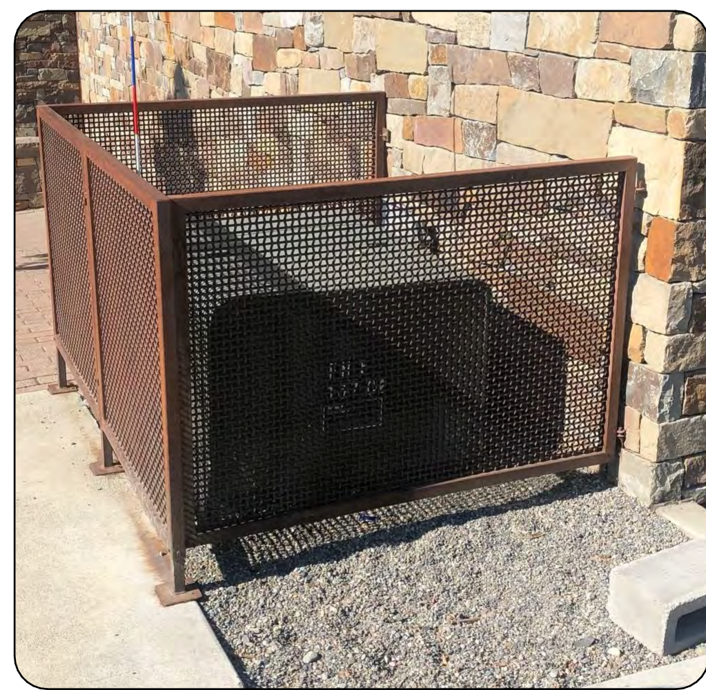
PHOTO: TRANSFORMER COVER EXAMPLE
