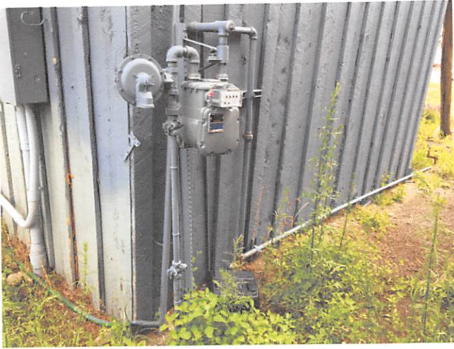
Existing Gas Meter
