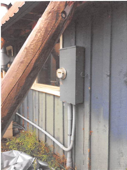
Main Electrical Panel
