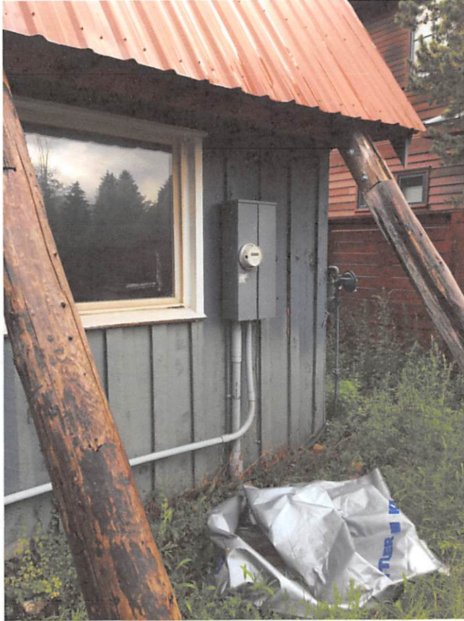
Main Electrical Panel
