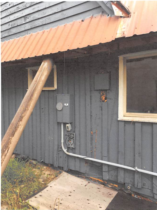
Existing Electric Subpanel
