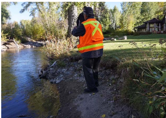
Figure 1: Eroding channel bank in project transition area.
