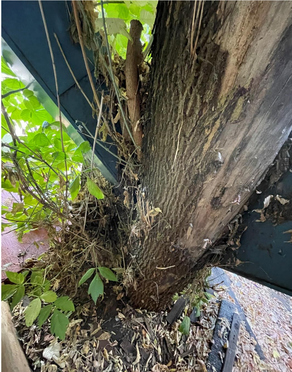
6. Tree Growth Compromising Foundation
