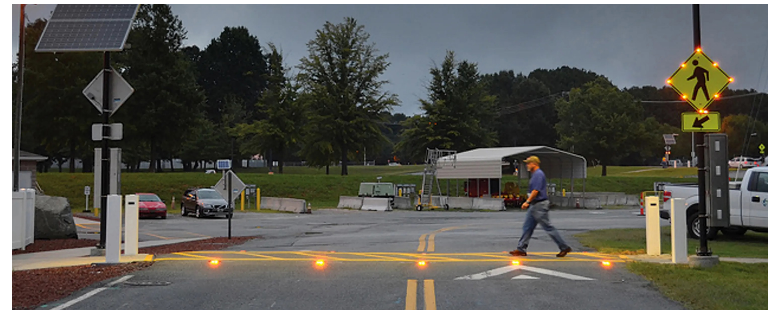
In Pavement Flasher
