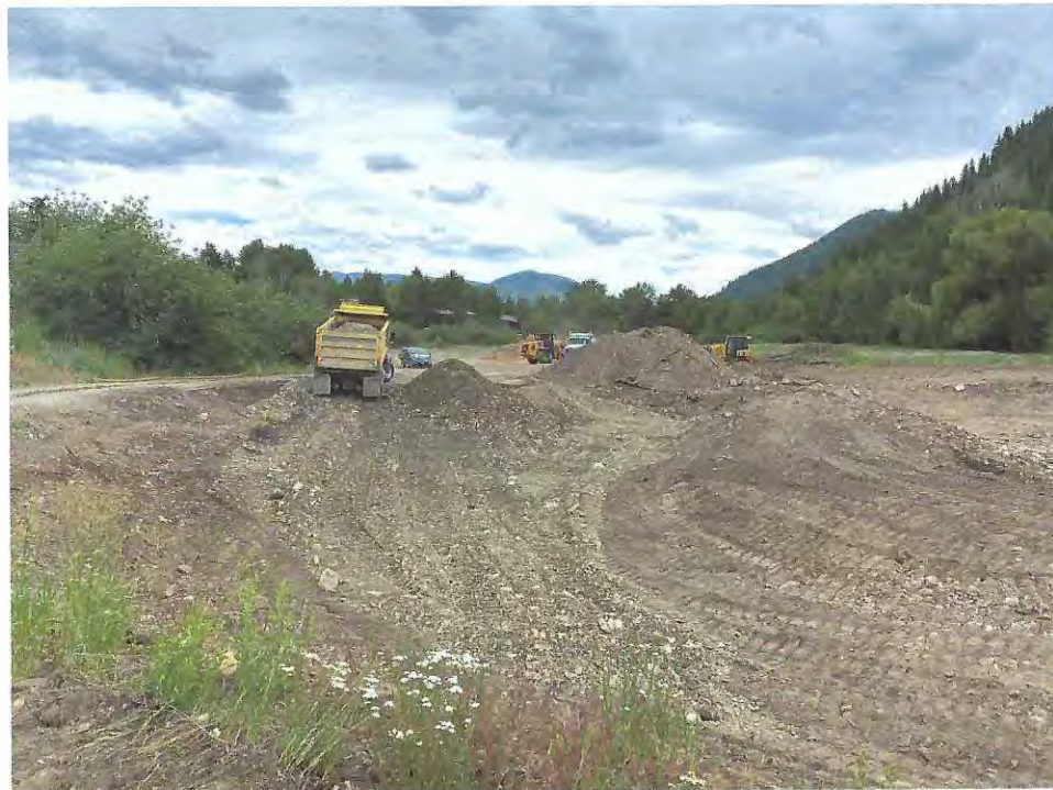
Imported sand and gravel being placed on compacted and approved native sand and gravel subgrade. 27Jun20
